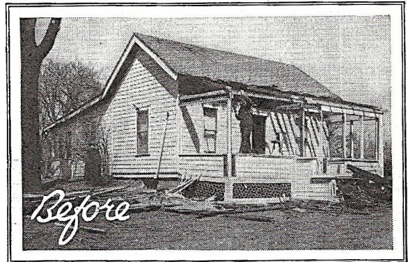
When re-roofing consider home revision. Photos show how addition improved ordinary cottage.
